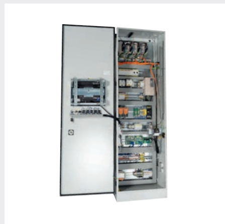
Electrical panel and control panel integrated in the machine frame
